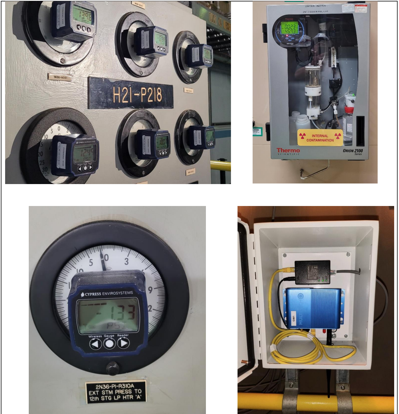
Figure 5 – Installation at Hatch - Operating Nuclear Power Plant
