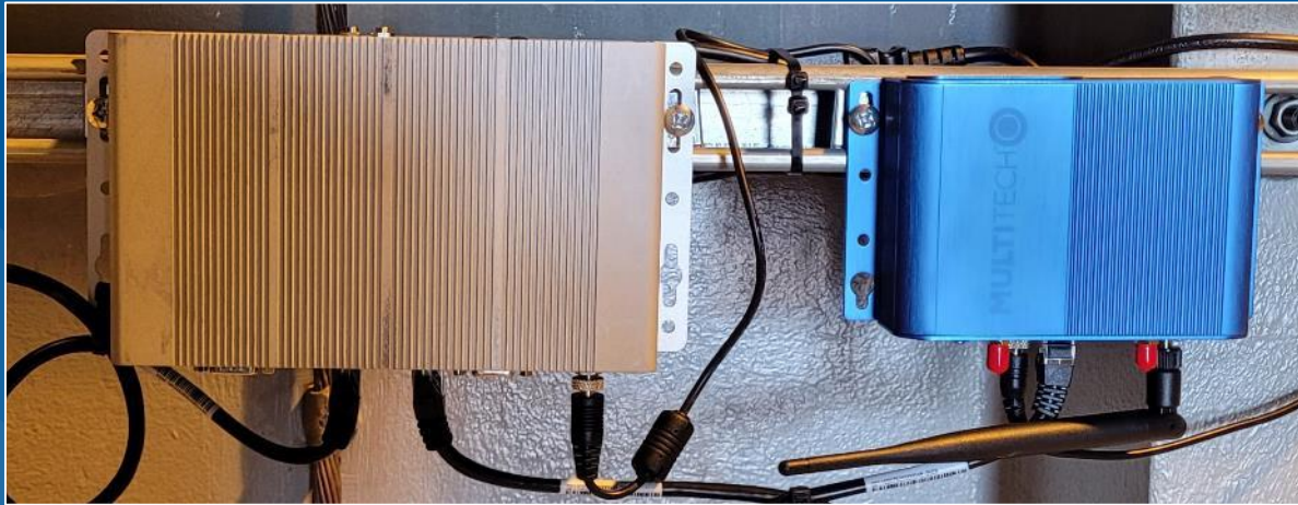
LoRaWAN Wireless Gateway and Controller
