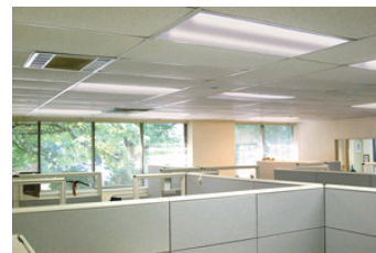
Legacy Fluorescent Lighting
