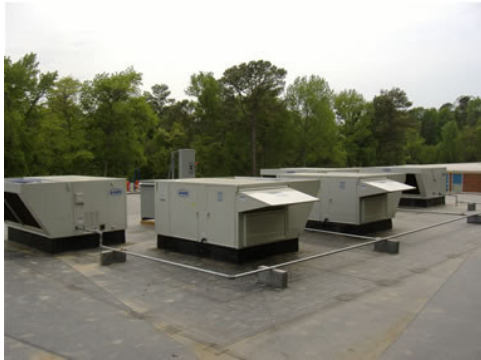
Typical Air Handler Units
