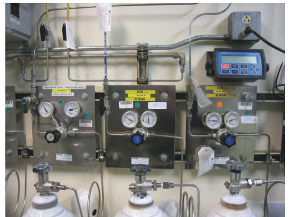
Figure 1. A typical Micrel gas cylinder area
