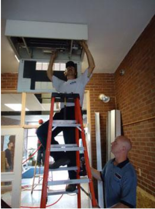
A Linc Mechanical technician installs cabinet heaters in one of the district schools.
