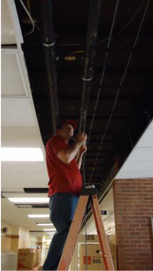
Drilling newly installed hot water piping in the ceiling at the high school.
